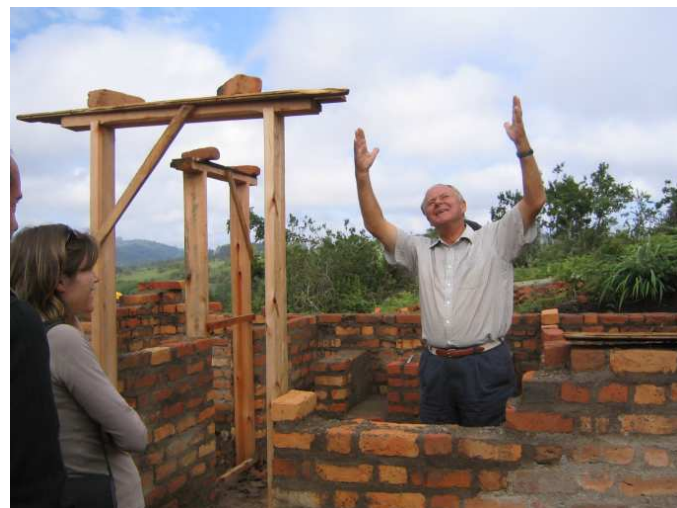
"Halleluiaah", says Geoff Fox, "At last we're underway". Visitors admire progress on the first orphanage building. Feb 2006
